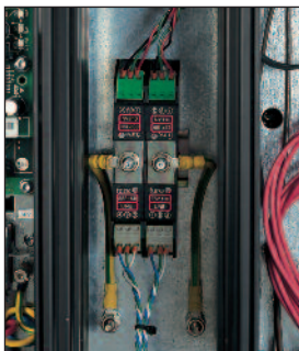
Two ESP 15H protectors mounted in a control cabinet and earthed via the cabinets' earthed chassis
