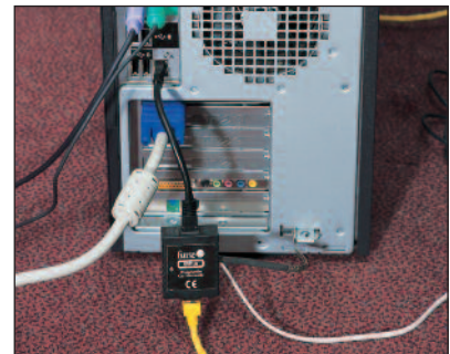
ESP LN installed on the network connection to a PC. Note the black earth lead connection to the chassis of the PC
